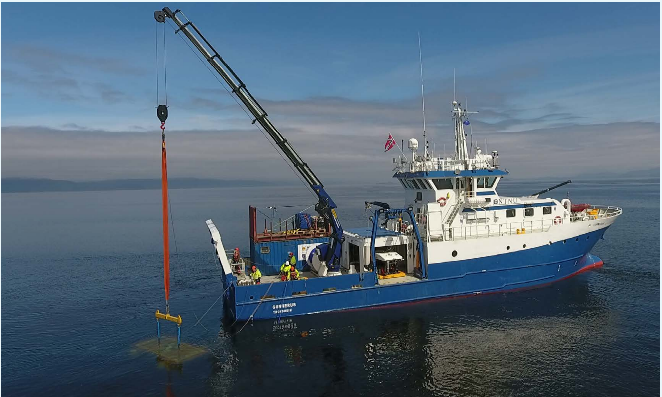
Centre for Autonomous Marine Operations and Systems (AMOS): The AMOS/NTNU-boat ‘Gunnerus’ during installation of Norway’s deepest underwater lab. © NTNU
